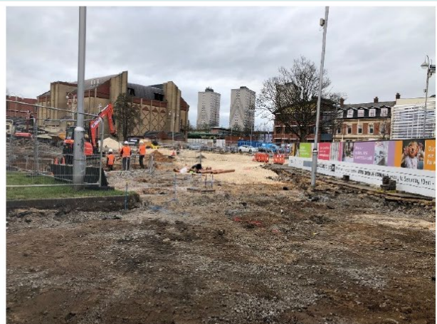
Photograph looking Westwards across site from 20-21 entrance. Drainage works and general progress shown
