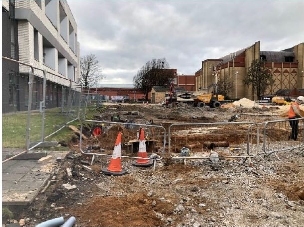
Photograph looking Westwards across site from 20-21 entrance. Drainage/gully connection excavation in progress (hand dig).
