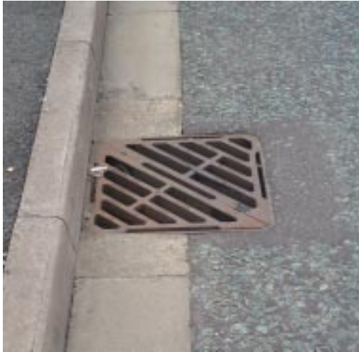
(left) - Ductile iron gully cover, draining a channel of pre cast concrete channel blocks. (Hot Rolled Asphalt carriageway)
