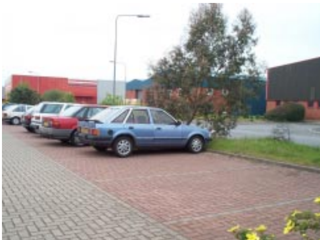
(left) - Concrete block paving used for the construction of a car park. Note the use of different colours to mark out the individual parking bays
